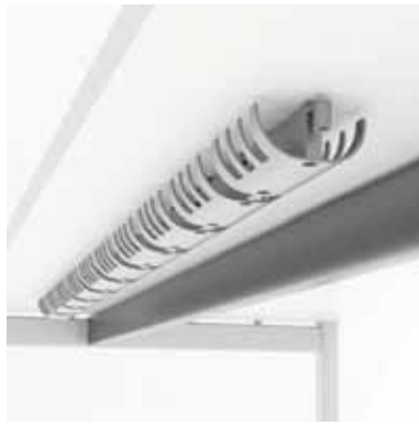
S82 CABLE RACK
